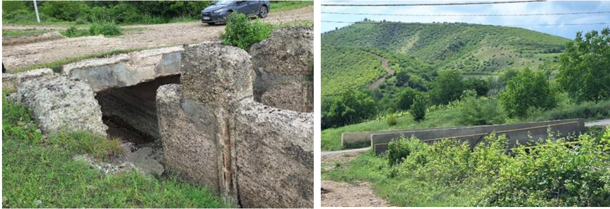
Figure 42. Existing rural bridges on the canal, located within the rehabilitation process transport corridors
