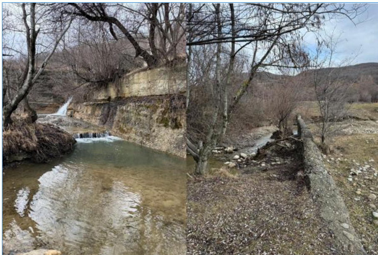
Photo 1: Existing scour and structural deterioration at the downstream side of the Narekvavi headworks.
