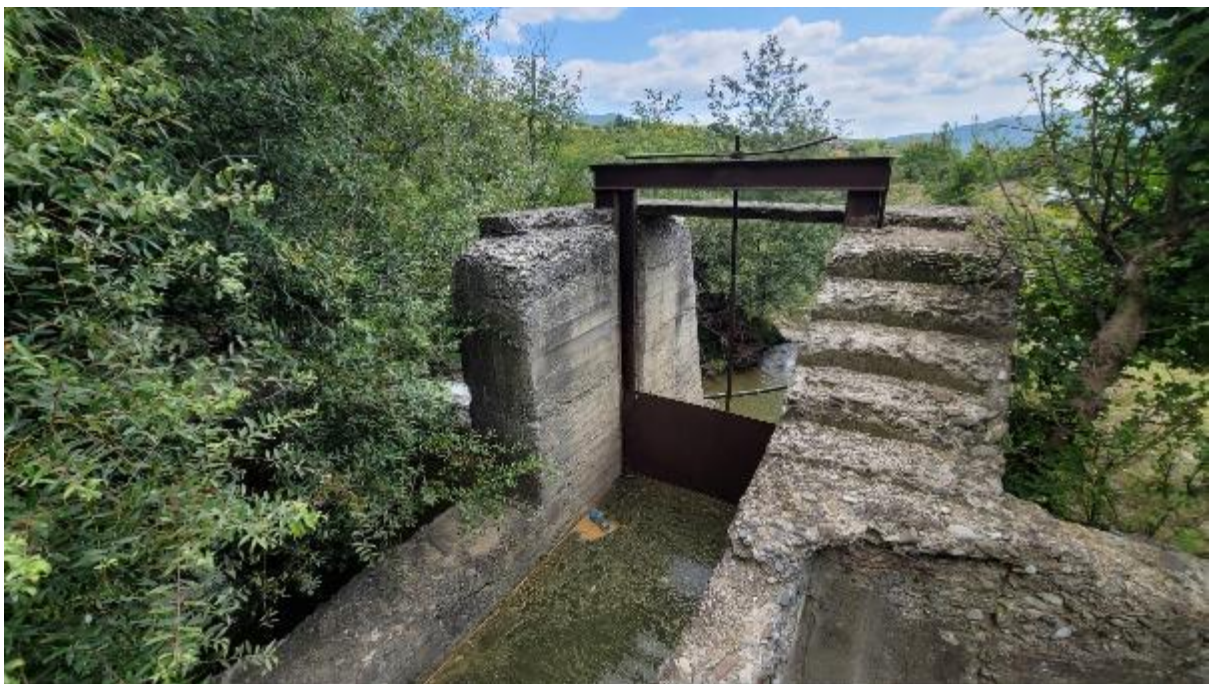
Water degradation due to water pounding in the existing scheme
